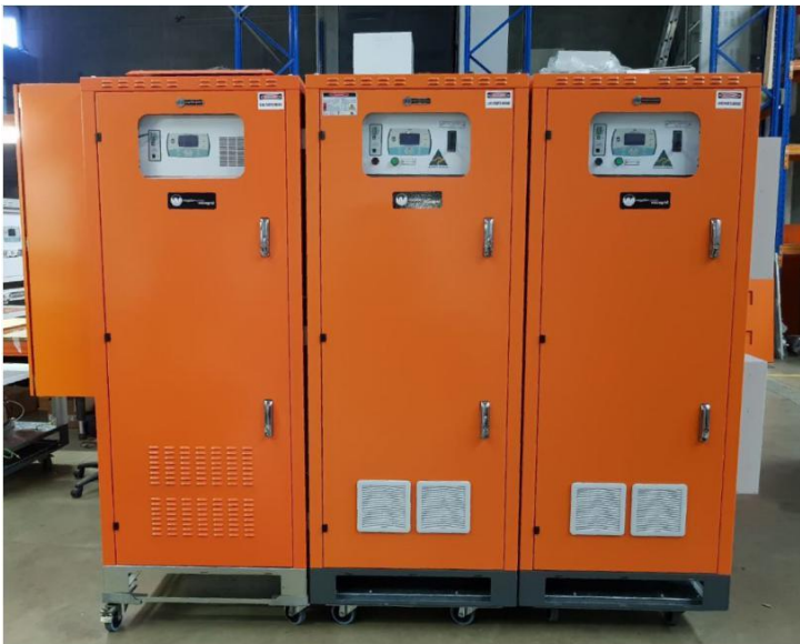
10kW inverter plus 35kWh battery bank
